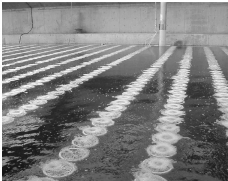
Fine Bubble Diffusers installed in 2001
